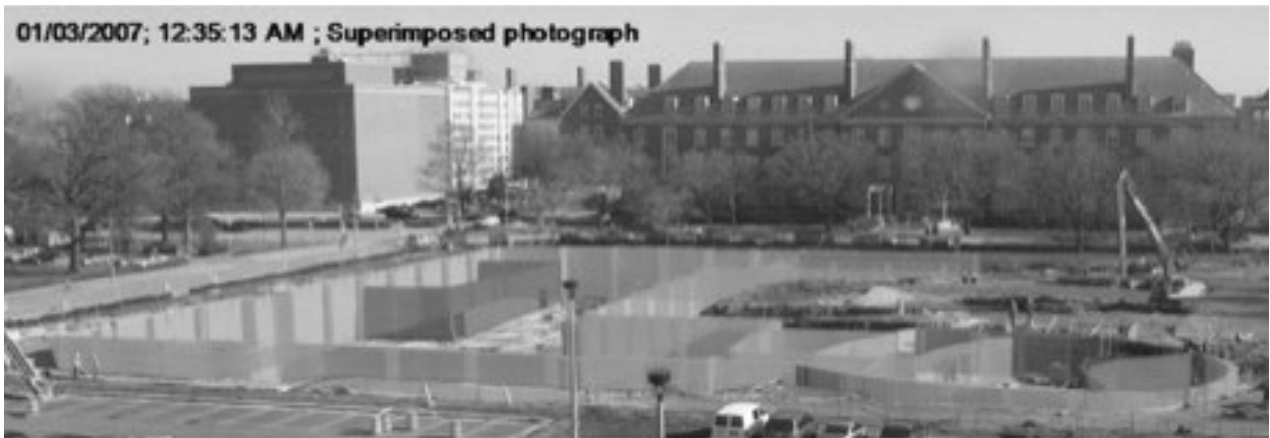
Figure 2 3D as-planned color coded model superimposed on the site photograph. (Source: Golparvar-Fard et al. [2], 2009)
